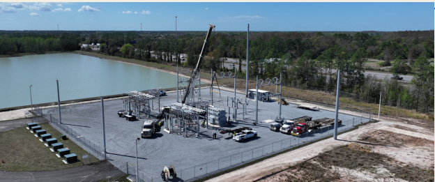
The Billy E. Brown Substation in Pasco County.
