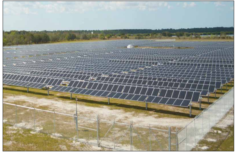
A view of our 2.2 MW solar farm in Hardee County installed in 2017.
